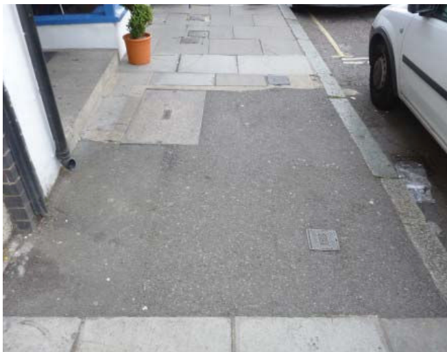
Inconsistent ground surfaces create an untidy and seemingly uncared for environment
